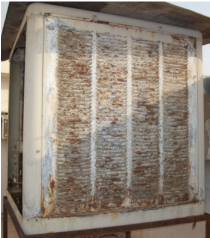
Fig. 2. The effect of the cumulated salt on the evaporative cooler (outside the cooler).
