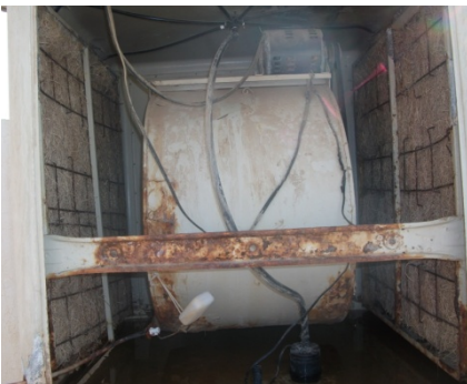
Fig. 3. The effect of the cumulated salt on the evaporative cooler (inside the cooler).
