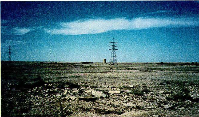
Fig. 22. A typical view of electrical transmitting lines. Metaphorically, they share other towers in carrying the electrical power.
